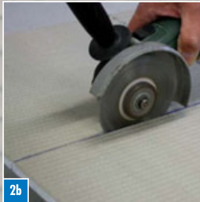
2b Apply the angle grinder (segmented diamond grindingsheet) and cut through along the cutting line (very easy cutting).
