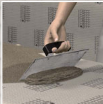
The application of fixing adhesive with a smoothing trowel is recommended e.g. as a contact layer.
